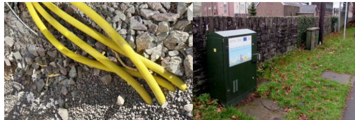
Fig. 2.5 (a) Underground cables (b) Telephone line junction box along the road
