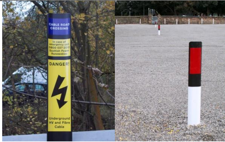
Fig. 1.14 Route marker and warning tape on the ground surface
