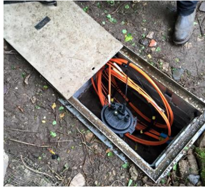
Fig. 1.11 Optical fibre cable kept in manhole in the form of coil
