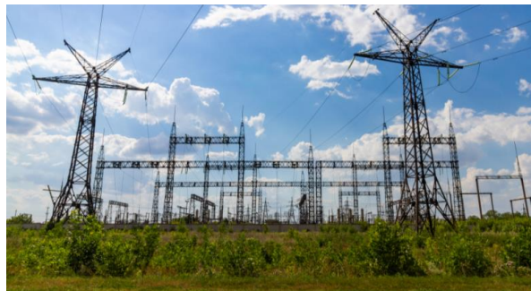
Fig. 2.20 Electrical substation and transmission tower
