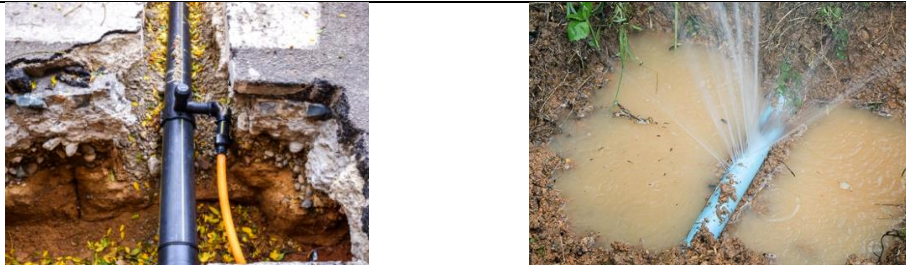
Fig. 2.10 (a) OFC close to water pipe (b) Water pipe damage in the excavation
