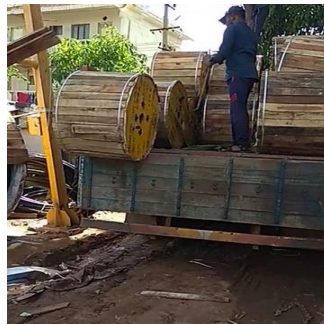
Fig. 3.8 Person is directly dropping the cable drum on the floor
