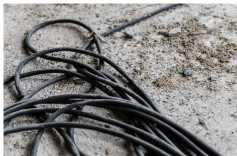
Fig. 1.7 Wrong way to put the optical fibre cable on the floor
