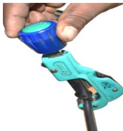
Fig. 3 Removing the jacket of the optical fibre cable using round tube cutter
