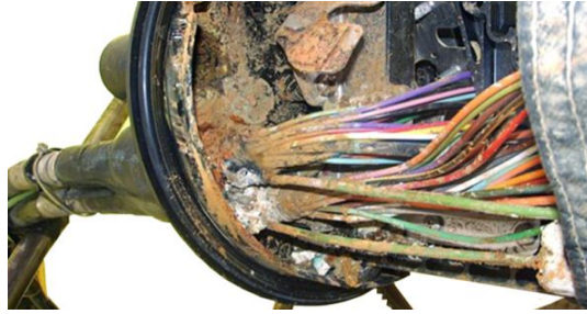
Fig. 2.3 Damage in the splice enclosure due to water
