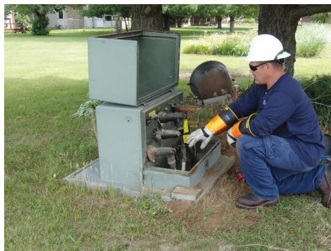
Fig. 2.21 Precautionary measures must be performed near the electric panel
