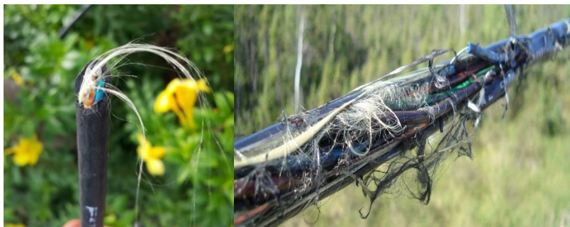
Fig. 2.2 Damaged optical fibre cables
