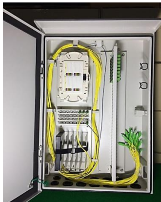
Fig. 1.26 Wall Mount Optical Distribution Frame
